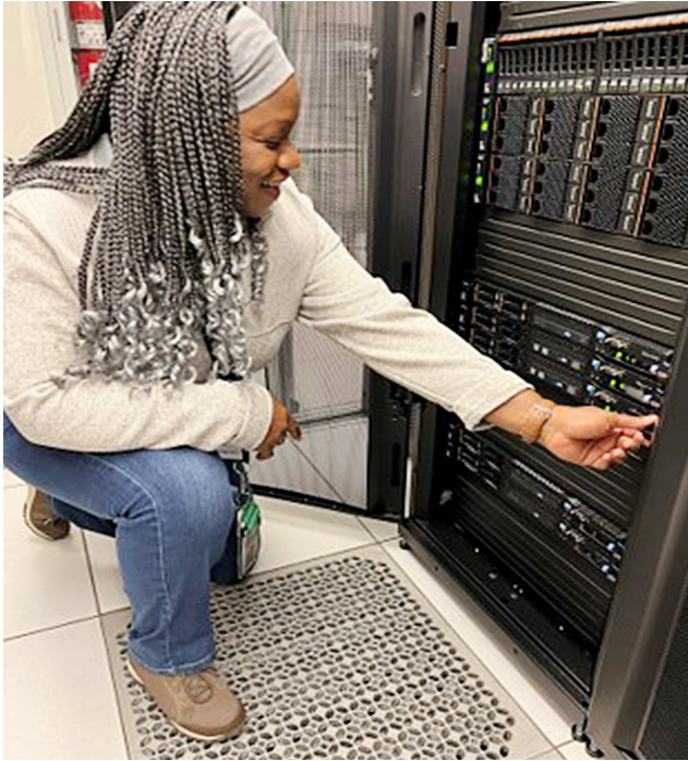
An L3Harris team member tests new server equipment at the Consolidated Backup. Photo credit: L3Harris
